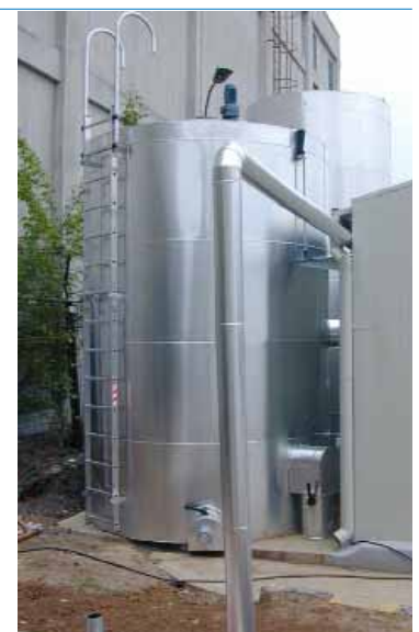
Sedimentationsbecken Sedimentation tank
